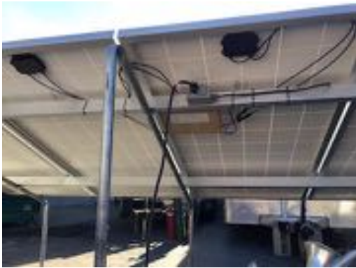
Inverter with power receptacle
