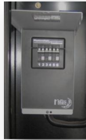
Figure 15 Combiner/ Breaker box, accessing breakers
