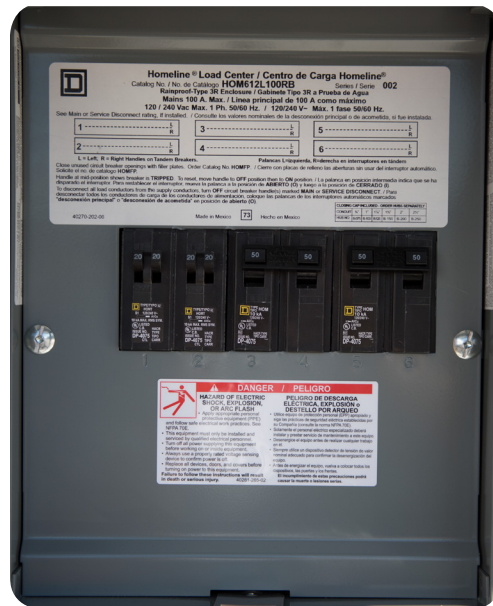
Figure 7 100 Amp Load Center
