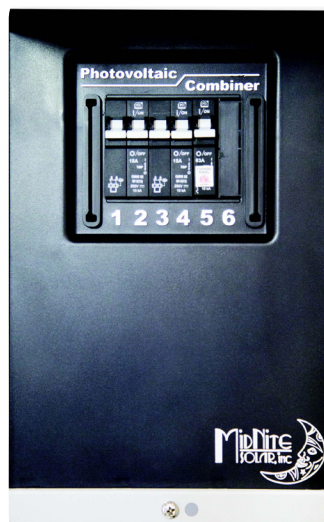
Figure 6 PV Combiner Box
